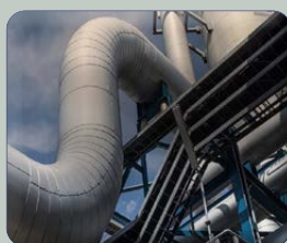
Examination and Simulation of Failure Analysis in 90-Degree Elbow Joints
